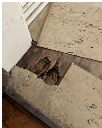
Close-up of hole in the flooring and asbestos tiles
