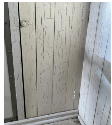
Close-up of cabinet condition and lead paint cracking
