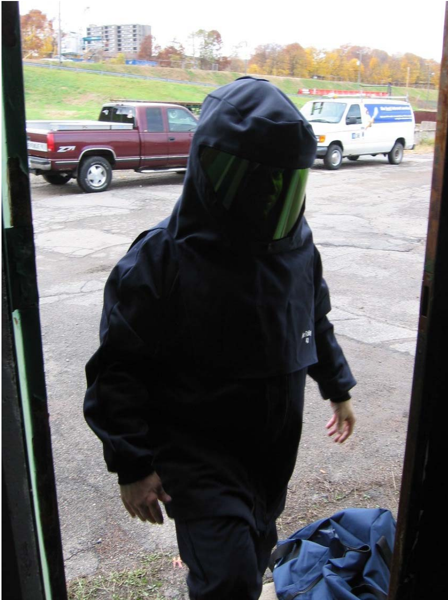
Flood Control Pump Station #1 Protective blast suit required to operate breakers
