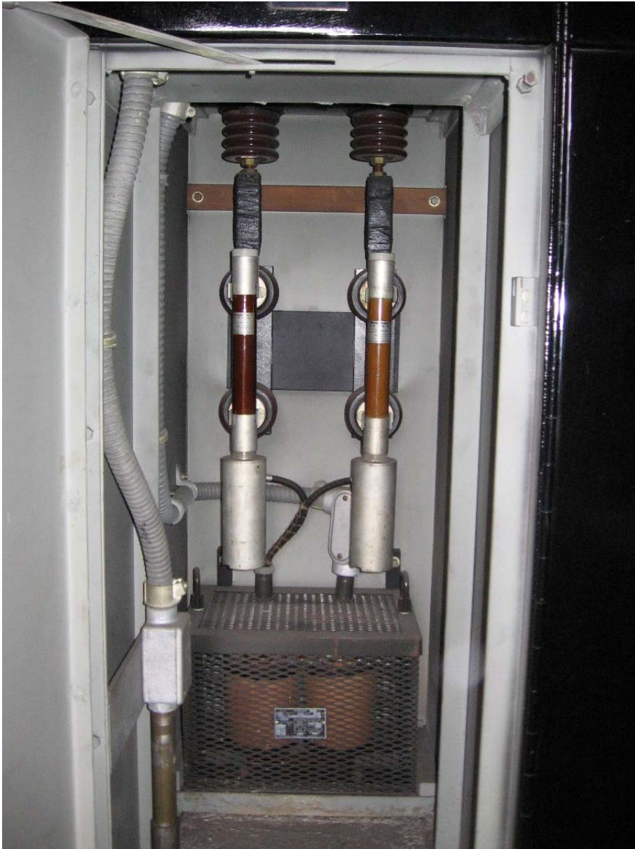
Flood Control Pump Station #1 Live front station service transformer
