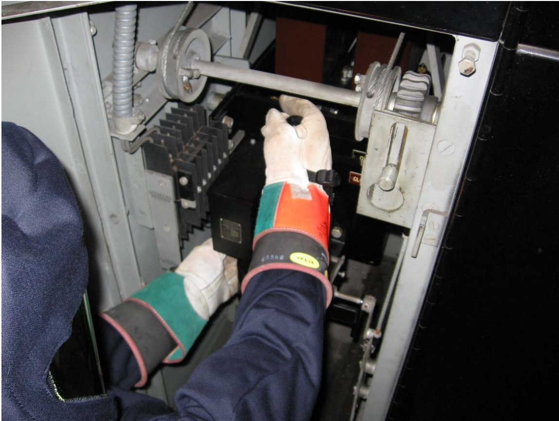
Flood Control Pump Station #1 Electrician preparing to close breaker
