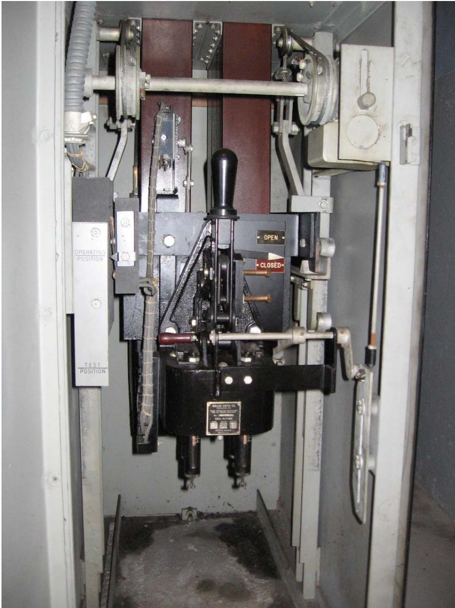
Flood Control Pump Station #1 Closeup of breaker
