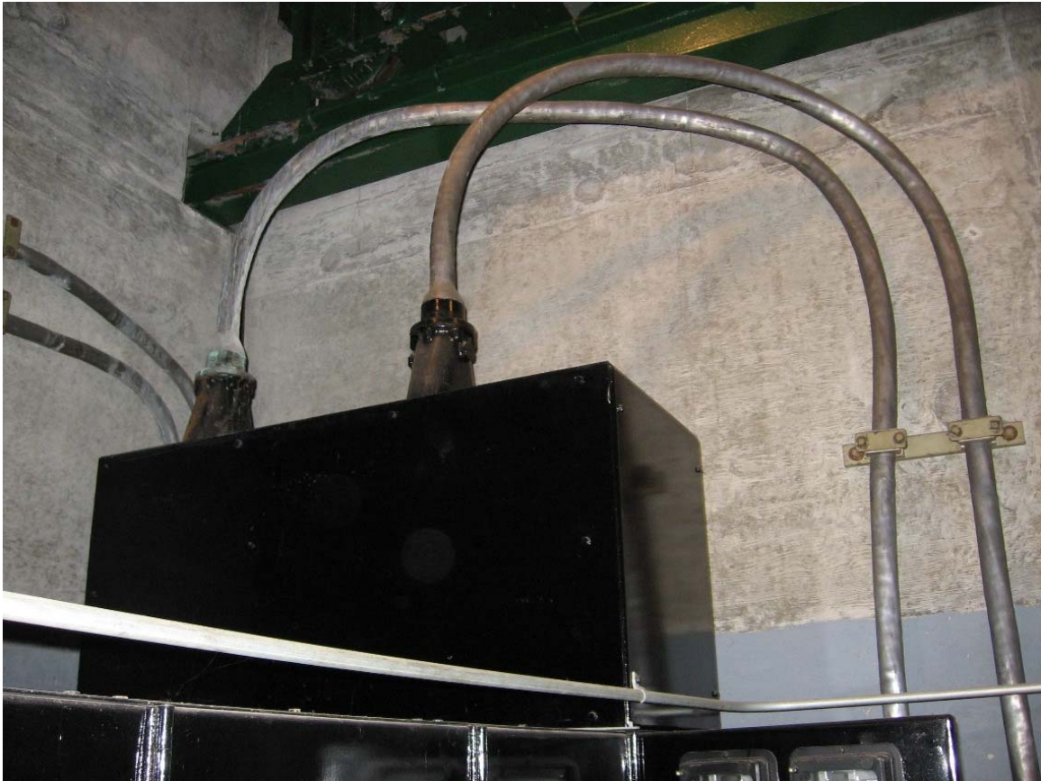
Flood Control Pump Station #1 Incoming lead cable
