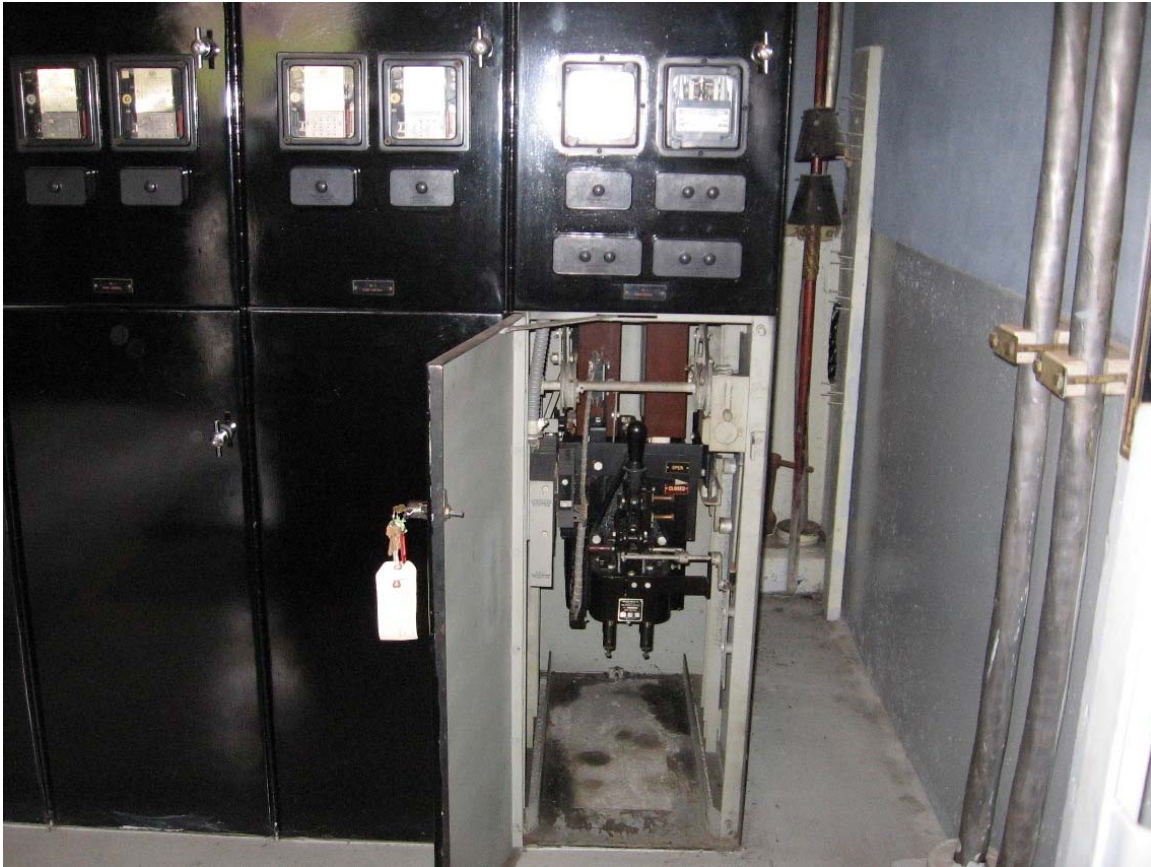
Flood Control Pump Station #1 Front view of switchgear lineup
