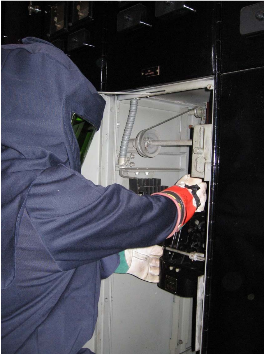
Flood Control Pump Station #1 Electrician preparing to close breaker
