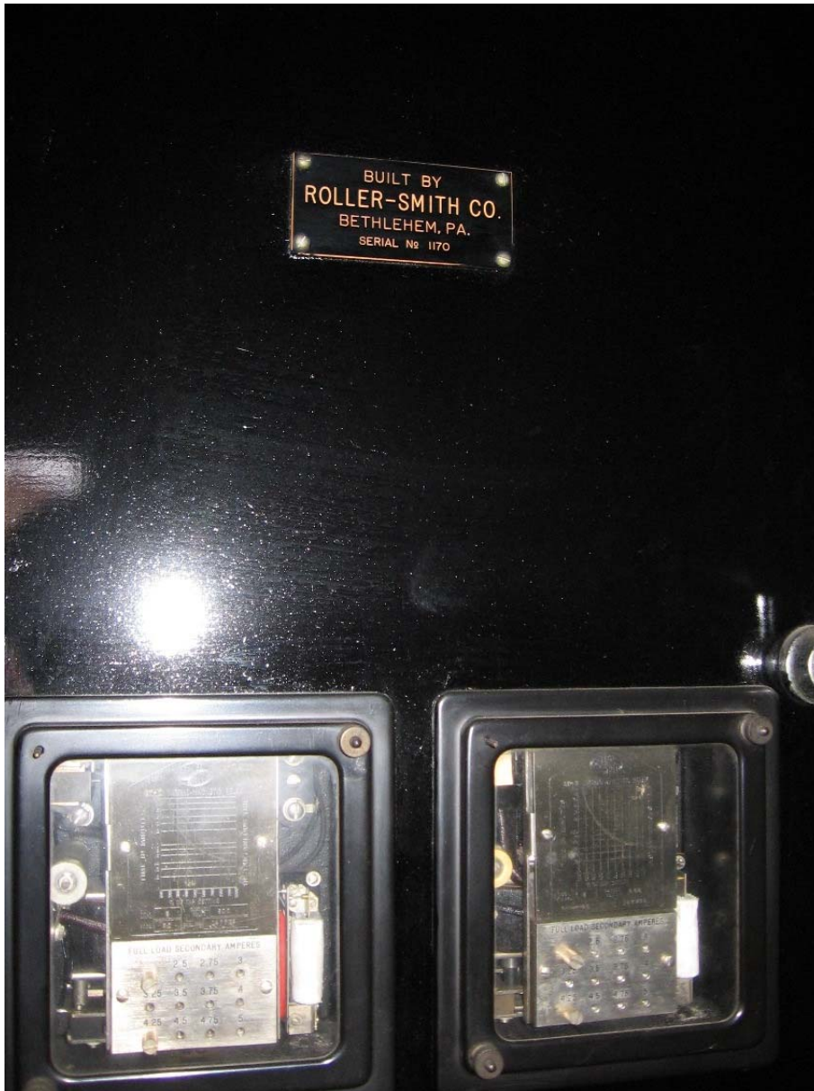
Flood Control Pump Station #1 Antiquated protective relays
