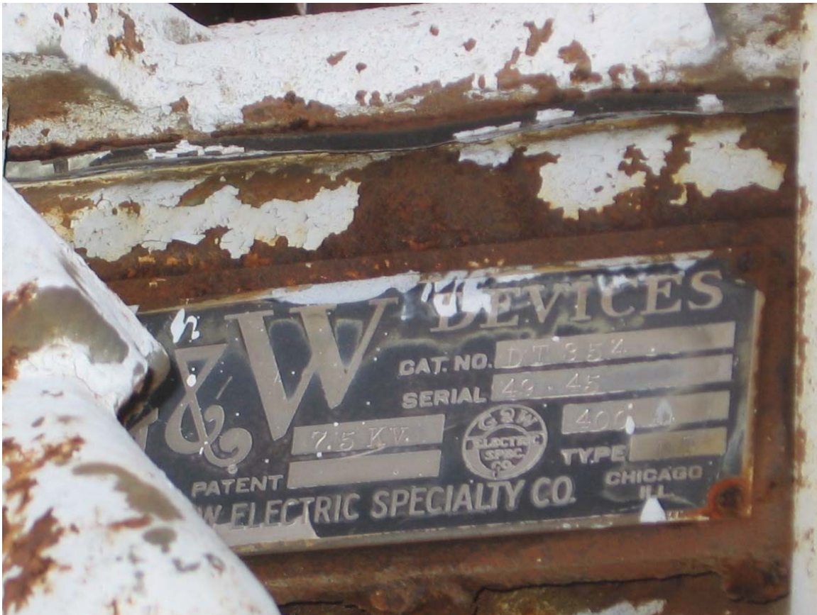
Flood Control Pump Station #1 Name plate for oil switch in substation
