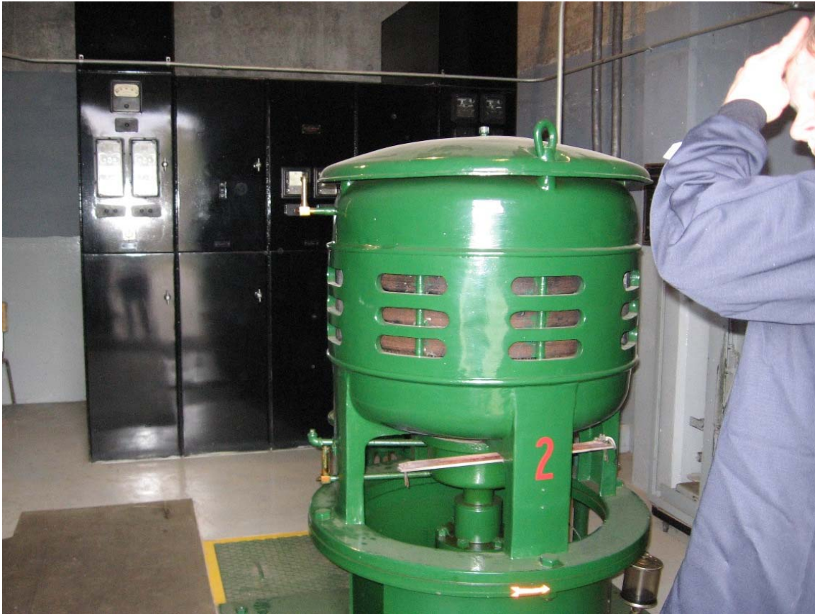
Flood Control Pump Station #1 Green pump and switchgear in background
