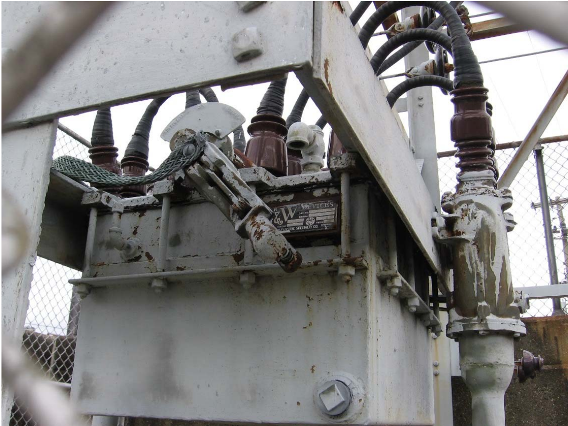
Flood Control Pump Station #1 Oil switch in substation
