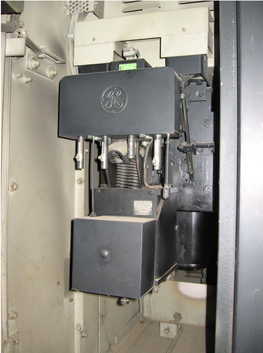
Flood Control Pump Station #7 View of Breaker
