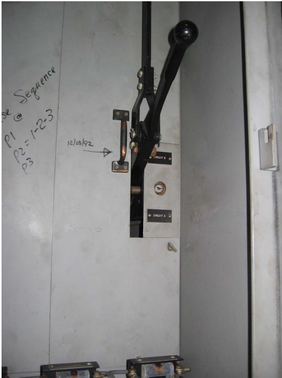
Flood Control Pump Station #1 Manually operated line disconnect switch operator
